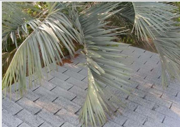
Trees Contacting Roof
