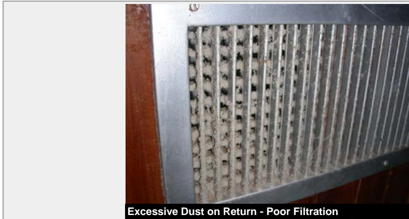
Excessive Dust on Return - Poor Filtration
