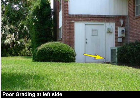
Poor Grading at left side
