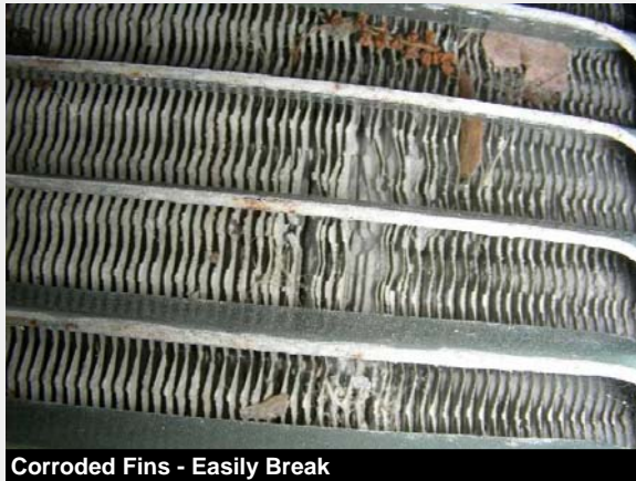
Corroded Fins - Easily Break
