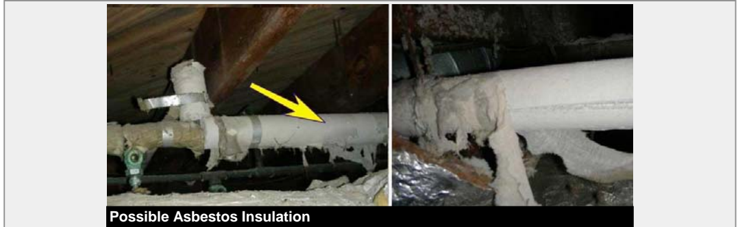
Possible Asbestos Insulation
