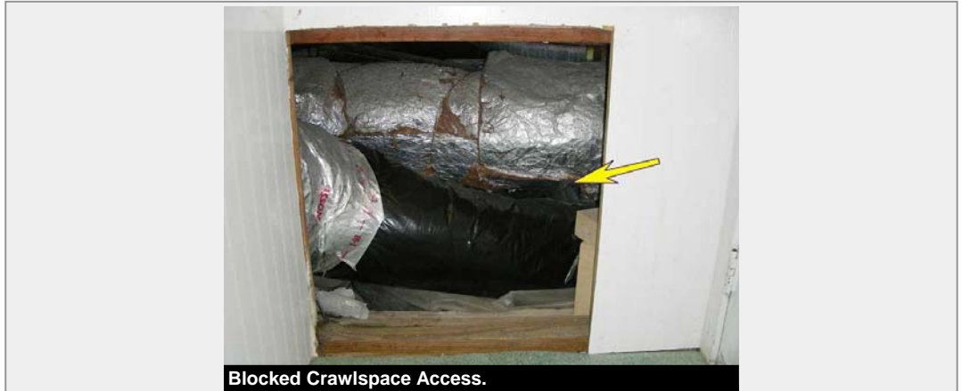
Blocked Crawlspace Access.
