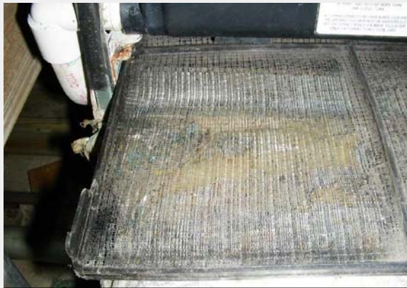
Thin ineffective Air Filter
