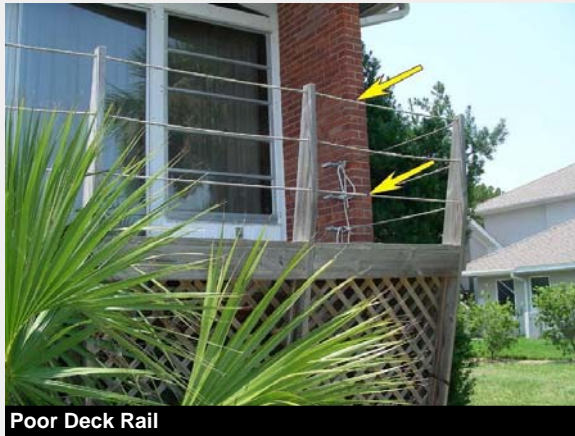
Poor Deck Rail
