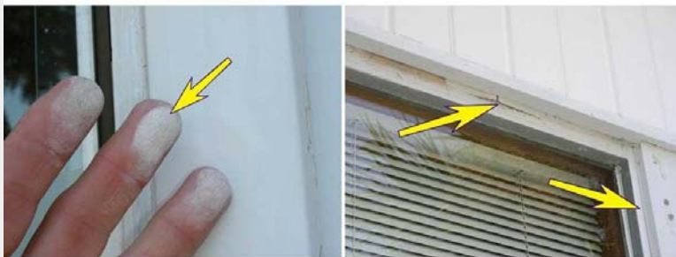
Worn Trim Paint / Sealing Needed at Joints
